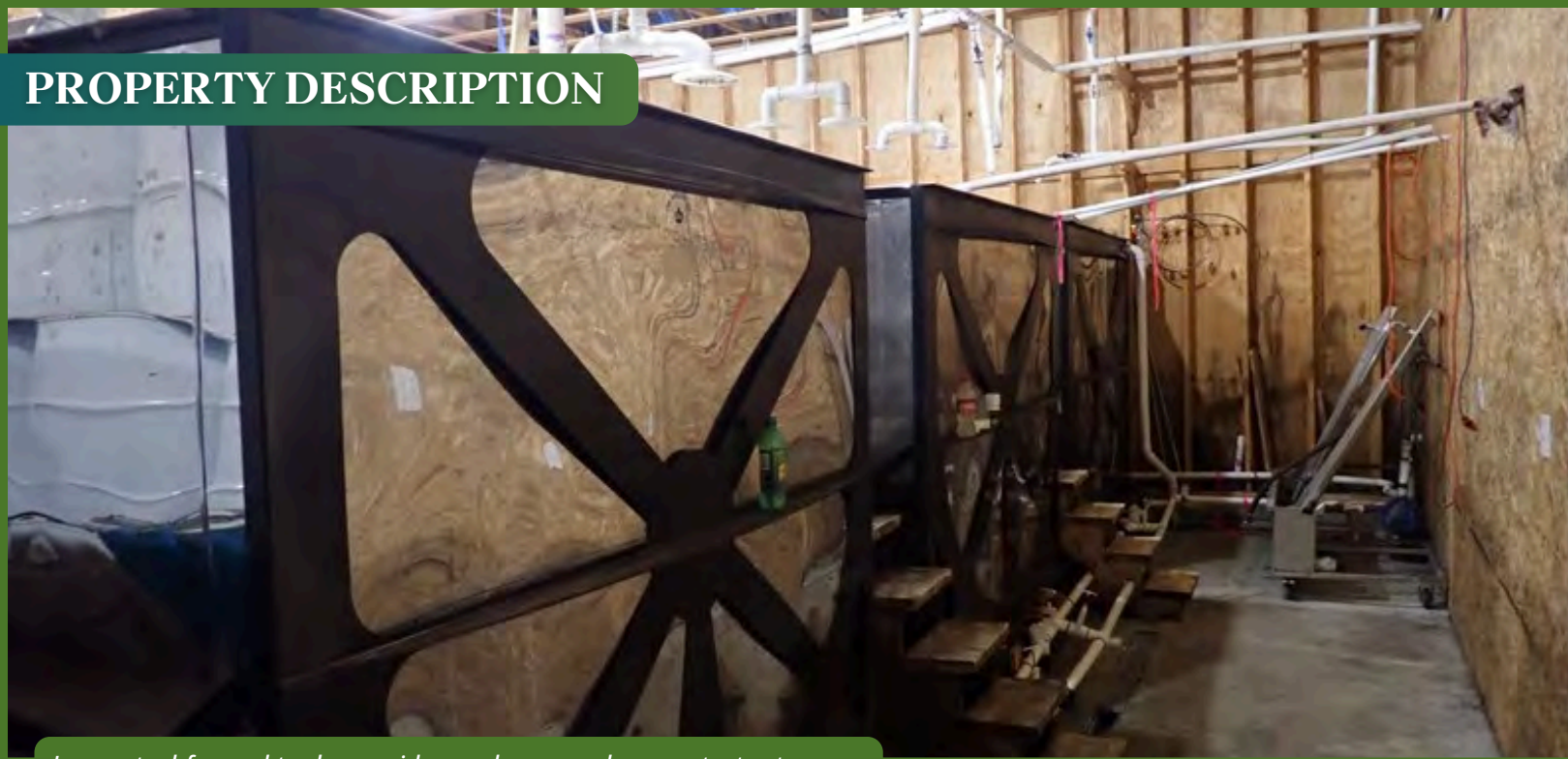
Large steel-framed tanks provide ample sap and concentrate storage.
