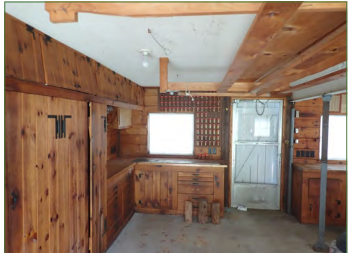
One bay of the garage was used as a workshop and has plenty of cabinets and benches in place.
